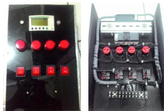
Gambar 3.4: Panel Kontrol Peraga Temperatur Ruang
