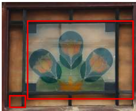
Figure 11. Ventilation of the Gedug Kembar
